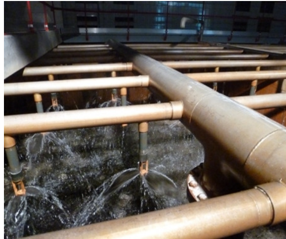
Figure 36: Spraying aeration on top of marble filter bed at Hoenderloo pumping station
